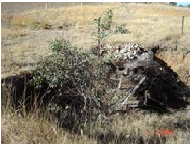
■ Figure 4-5 erosion head on G1/3
