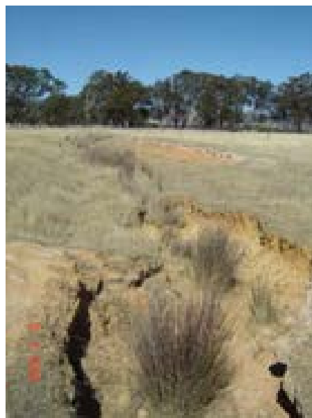
■ Figure 4-4 SCA style works on G1/2 require maintenance to secure ongoing integrity
