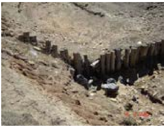
■ Figure 5-1 Failing pile field on S1
