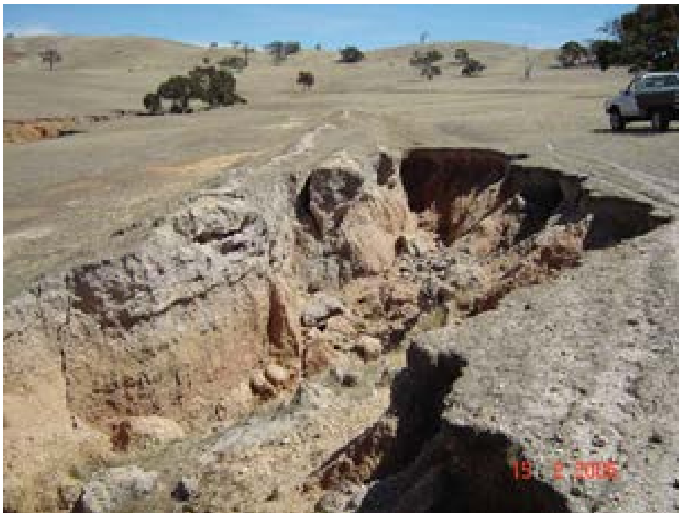
■ Figure 4-5 Failed diversion levee on S1/5 has resulted in major erosion
