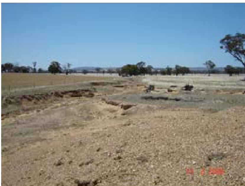
■ Figure 7-5 Channel incision and erosion along W6.1/2
