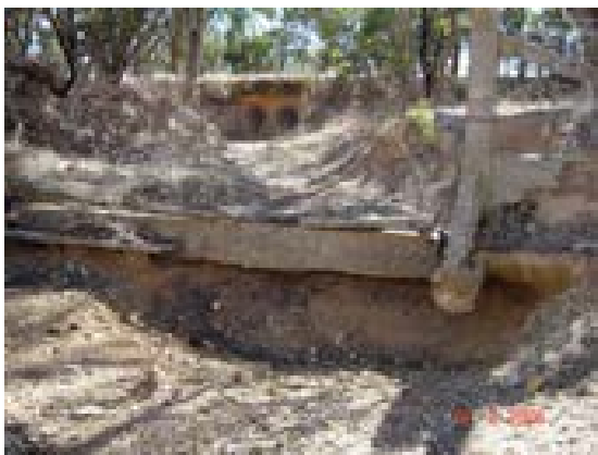
■ Figure 6-3 headward erosion on W5/3/1/1 is undermining existing structures
