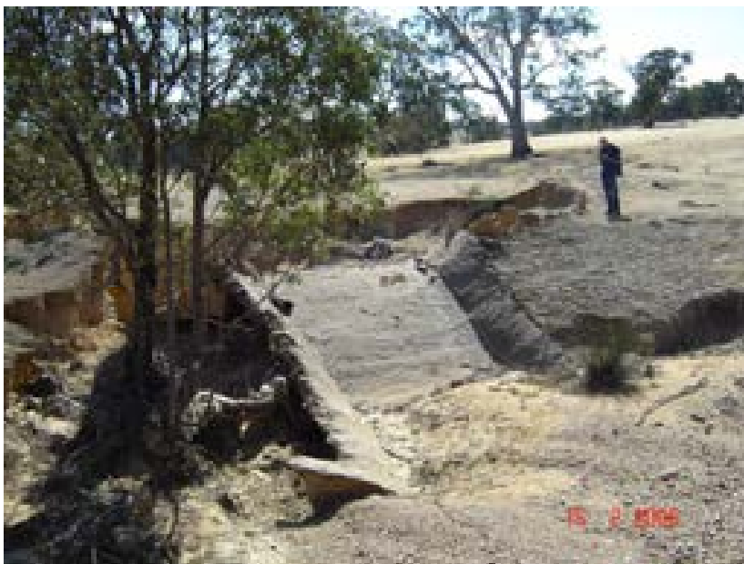
■ Figure 6-5 SCA style concrete chute on W5/4/1 has failed
