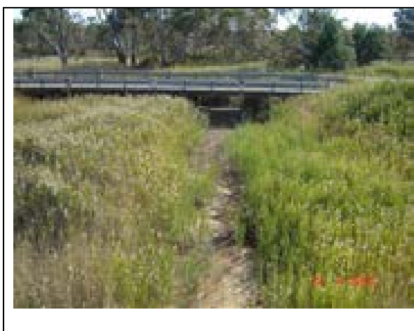
■ Figure 4.2 – Potential Flood danger at the Pyrenees Highway at the change of grade in Mt. Cole Creek
