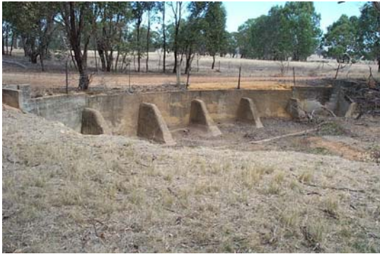
Figure 13: Structure on tributary of Seven Mile Creek at the corner of Martins Road and Potters Road
