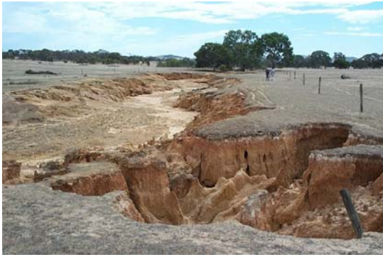
Figure 2: Active erosion head in Reach 2
