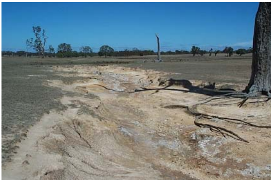
Figure 4: Salt affected creek in mid section of Reach 2
