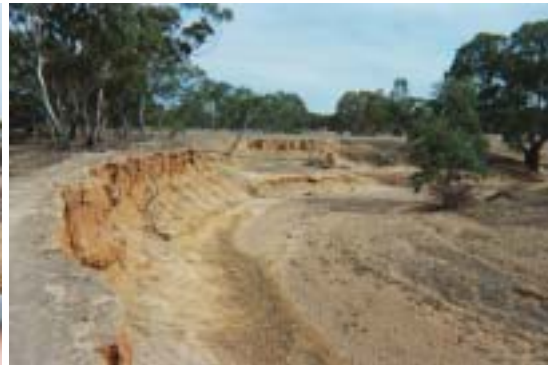
Figure 10: Outer bank erosion on Seven Mile Creek threatening Potters Road
