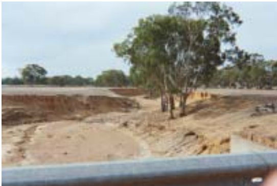
Figure 9: Over enlarged channel of Seven Mile Creek downstream from Vineyard Road
