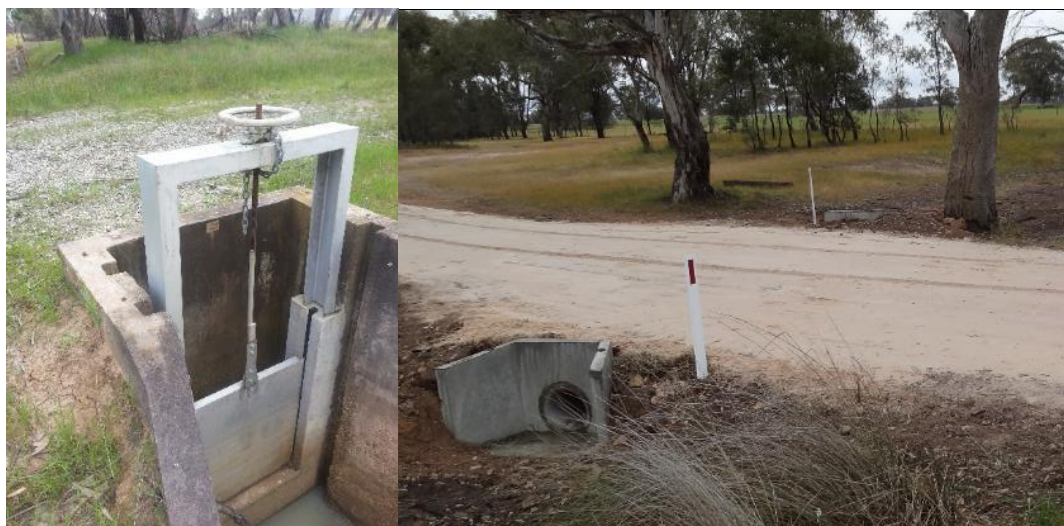
Figure 3-23. Bungalally Creek Regulator at Toolondo Channel (left) and low level crossing on the Bungalally Creek (right).
