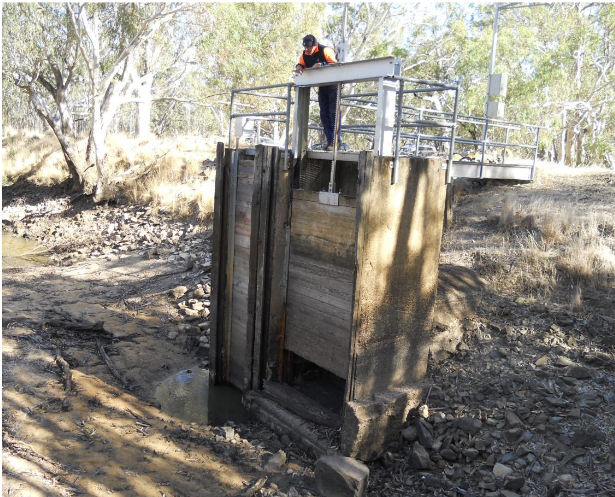
Big Pipe Outlet from the Wimmera Inlet Channel into the Wimmera River, May 2015
