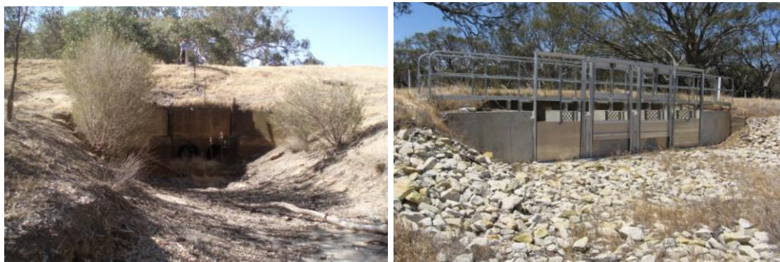
Figure 3-18. Example features that influence flows down Yarriambiack Creek such as the Yarriambiack Creek Offtake Regulator (left) and Brim Weir (right).
