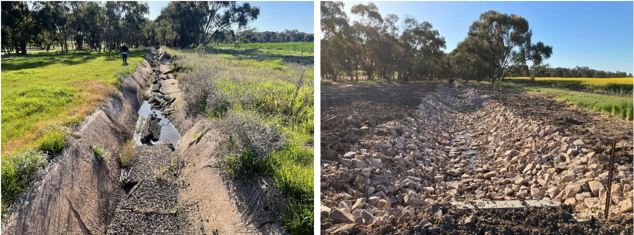
Figure 5-20 Upper concrete lined section of channel, before and after replacement with rockwork
