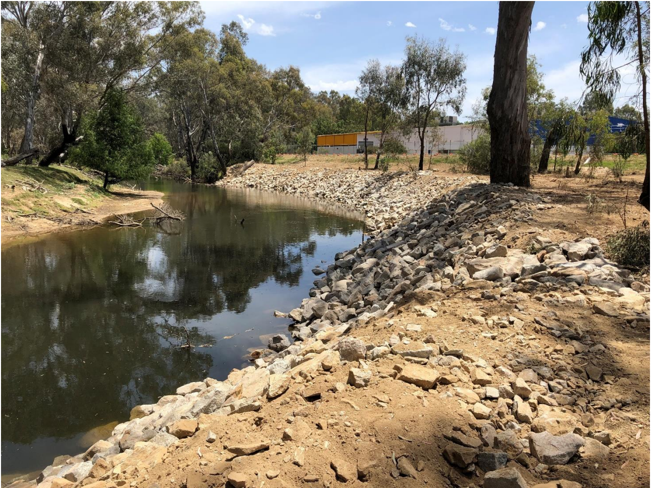
Figure 7-1 Rock beaching installed on the Ovens River at Wangaratta aimed at protecting an existing levee.
