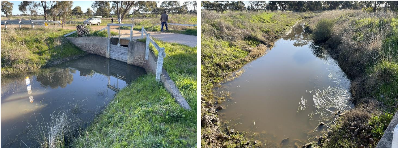
Figure 5-18 Offtake penstock gate and earthen channel immediately downstream.
