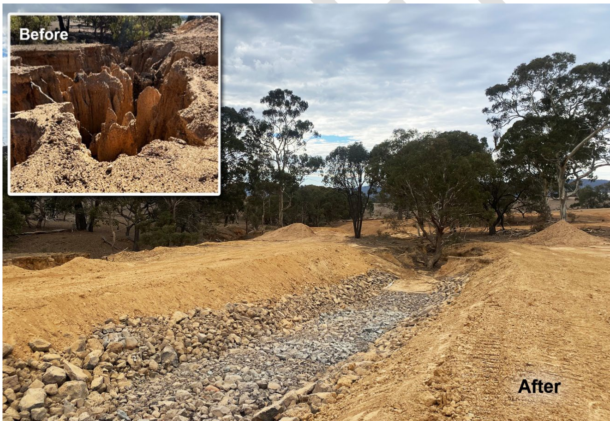
Works completed in an Upper Catchment waterway to reduce sediment movement and impacts downstream.
