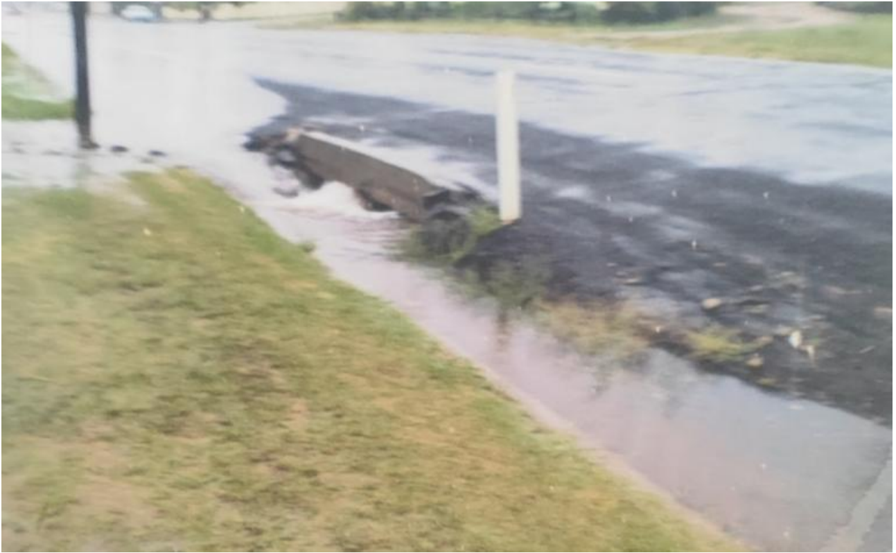
Figure 5-6 Flooding at Wallace Street Crossing
